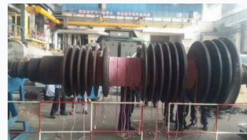
Rotor Bending Straightening
